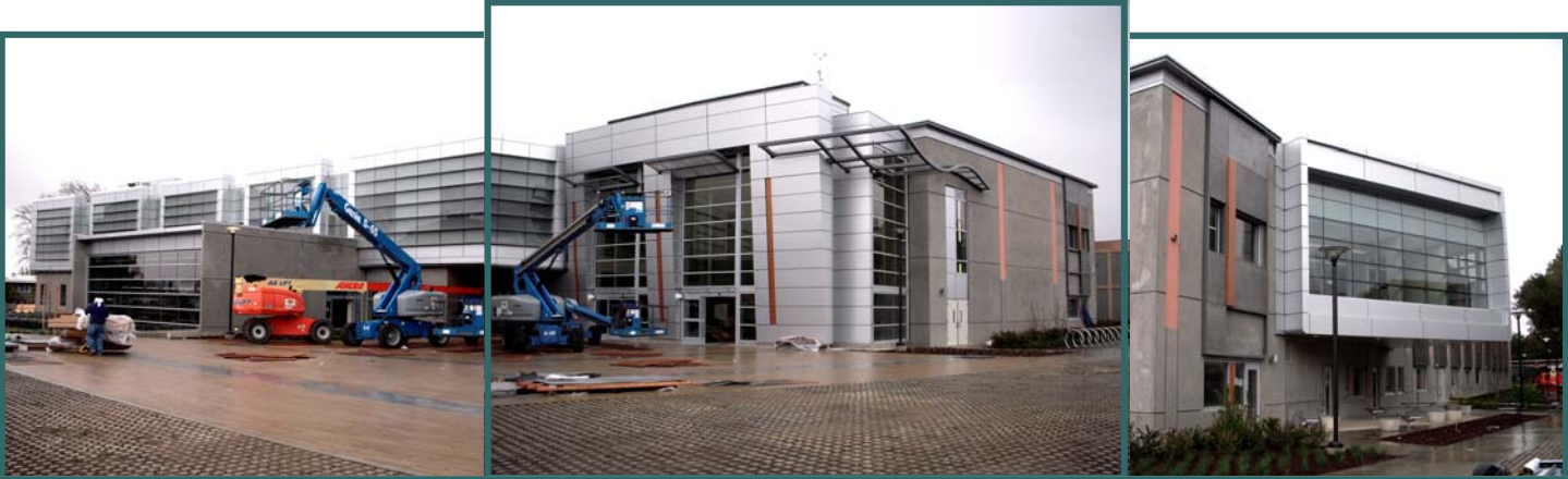
Front views of New CSSC Building still under construction. Photos courtesy of Isabel Braunstein
